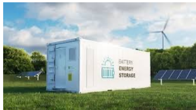
Battery storage: 2-4 MWh, 2 MWp
