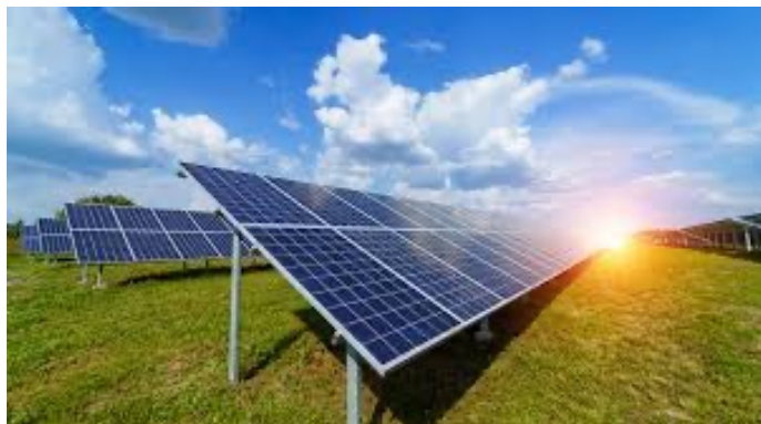
Solar PV: 7.2 MWp
