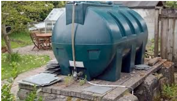
Oil and gas heating systems
